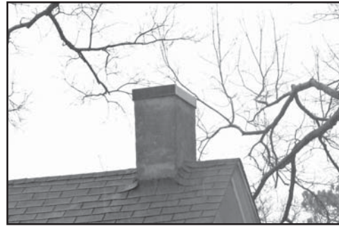
This interior chimney is covered in stucco. Stucco shall never be applied to a masonry chimney unless it was a historic feature of the building. If stucco was originally on a chimney it must be maintained.
