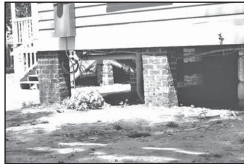
Original pier foundations must be maintained year round, and retained during any rehabilitation project.
