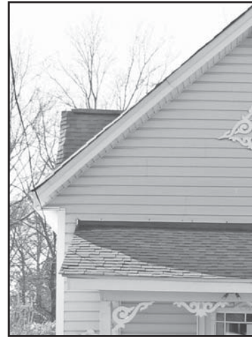
Wood clapboards, if maintained, can be retained indefinitely. When needed the replacement of portions of historic clapboards can be done in-kind. The covering of intact clapboards is not encouraged.
