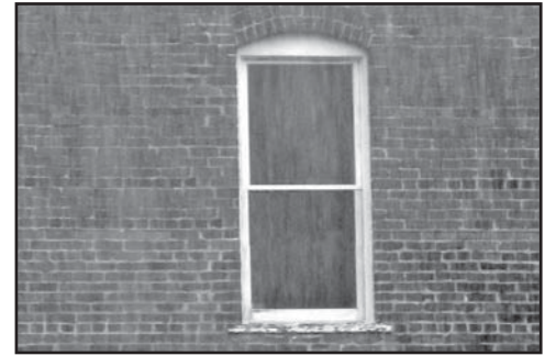
This original arched window opening is character-defining and must not be infilled or altered during rehabilitation of the building.
