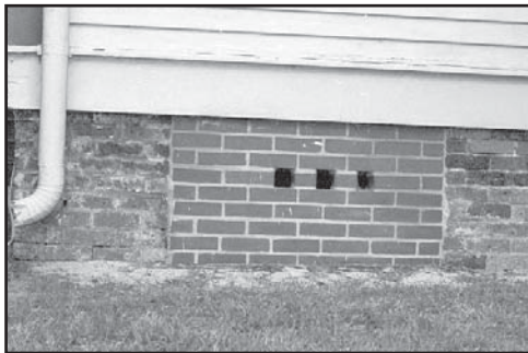
The solid infill of historic pier foundations is not encouraged. If they are to be infilled the new material must be stepped back from the front face of the foundation. When possible an open, lattice-like infill is suggested.
