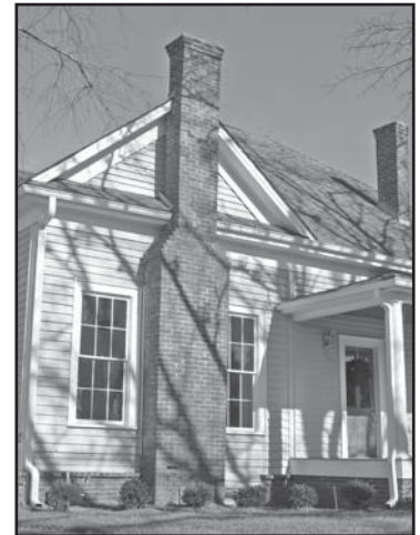
This gable end chimney is integral to the house type classification of this property. Its removal would effect the integrity of the property. Chimneys like this must always be maintained and must be retained during rehabilitation projects.
