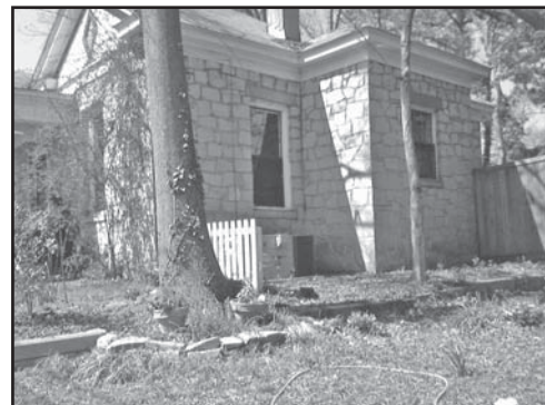
This HVAC unit has been screened by a picket fence. This is an appropriate solution to utilize when screening such mechanical services, although in this case the fence should have wrapped around this unit.
