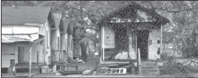
This shotgun house type in Columbus, Georgia, was abandoned and is in the process of demolition-by-neglect. Demolition-by-neglect attracts vandals which often may lead to arson, as in this case, which can easily destroy a whole historic area.
