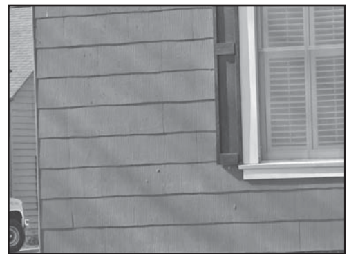
These asbestos shingles found in the Cherokee Street Historic District have achieved historic significance for this property and must be maintained and retained in future rehabilitation efforts of this property.
