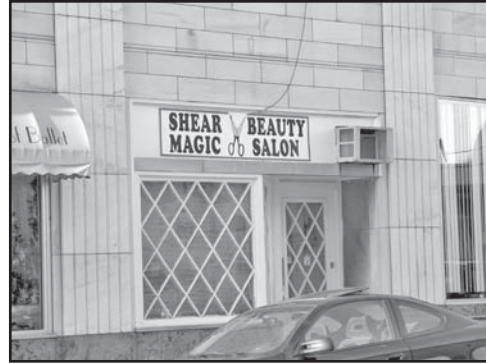
The placement of air conditioning units on the front facade of buildings is not appropriate. Such mechanical systems must be placed on facades not visible from the public right-of-way so they will not disrupt the historic integrity of the property.
