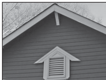
The vernacular roof brackets and attic vent are simple details on this turn-of-the-century cottage that are character-defining and must be retained.
