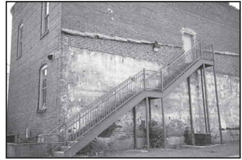
This simple and effective fire escape has been appropriately placed to the rear of this building.
