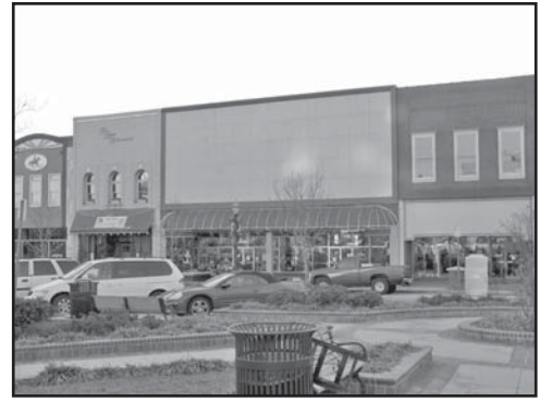
This storefront and upper floor in Gainesville, Georgia, has been inappropriately remodeled so that the original entrances have been lost and the upper floor windows have been obscured.
